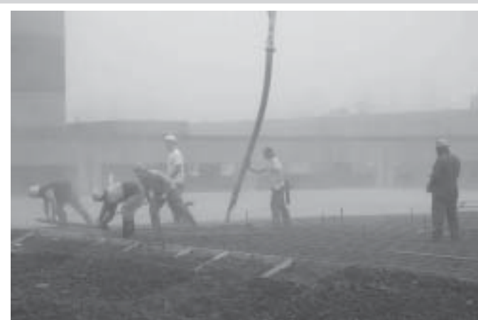
Construction of North Santiam building begins as workers lay the foundation on a foggy January morning. Additional photos of the ongoing construction can be viewed at the Capital Planning website.
