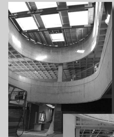
The open atrium area outside the bookstore will soon be replaced by a courtyard with an enclosed ceiling housing six skylights (left). HOWE (below) and the bookstore (bottom) are in the final stages of completion.
